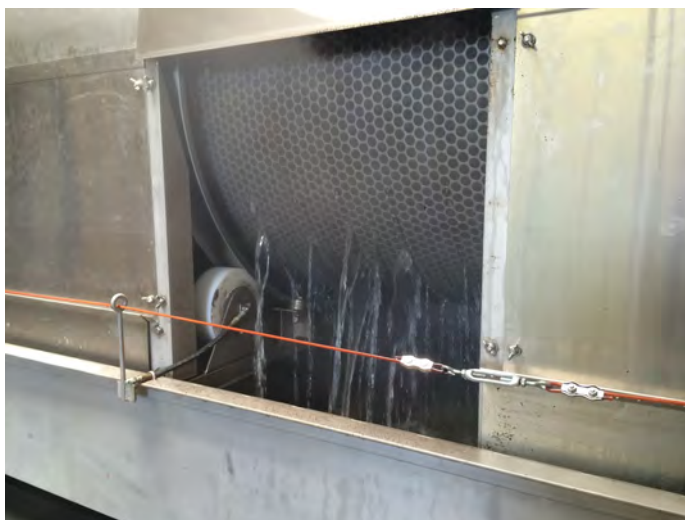
Figure 6-5: Side View of Drum Screen Inside a Rotary Drum Thickener
