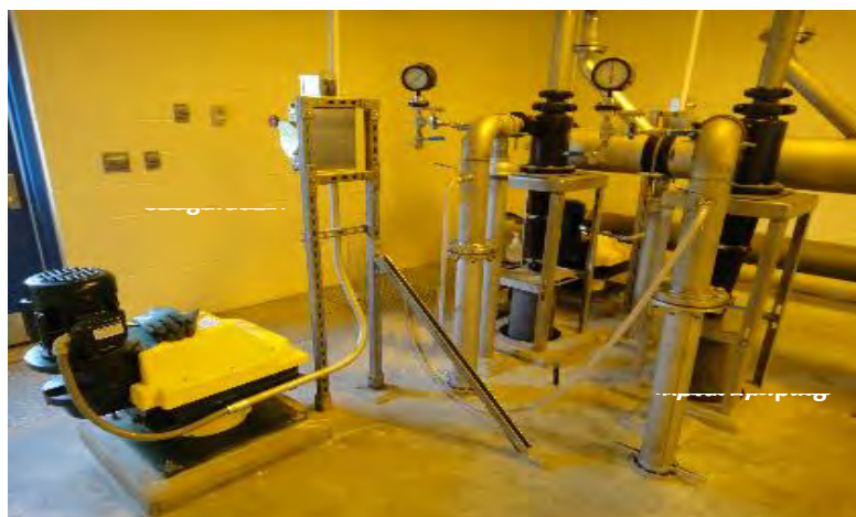
Figure 5-9: Actiflo Equipment at the Webster, MA WWTF
