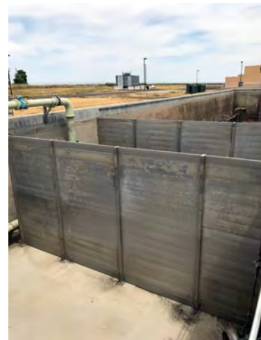
Figure 4-13: Baffle Walls in Anoxic Zone
