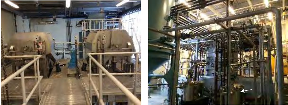
Figure 5-11: Magnetite Recovery Drums over Ballast Mix Tank (left) and Shear Mills (right) at the Marlborough Easterly WWTF
