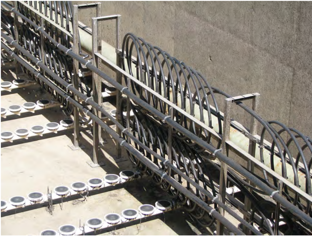
Figure 4-15: Heat Exchange Coils in the Aeration Basin
